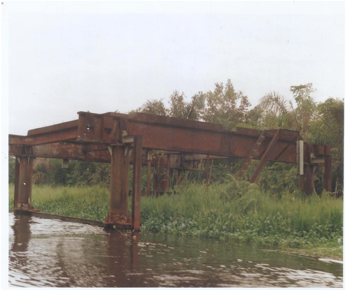
Figure 4.23: The Abandoned Platform of Shell at Biagbini, Arogbo, built in 1959.
