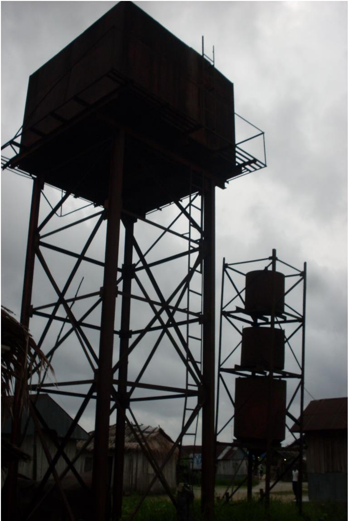
Plate 4.21: NAOC huge pipe borne water storage tank project under construction in Obuguru community, Ogulagha Kingdom. Source: Fieldwork, 2017
