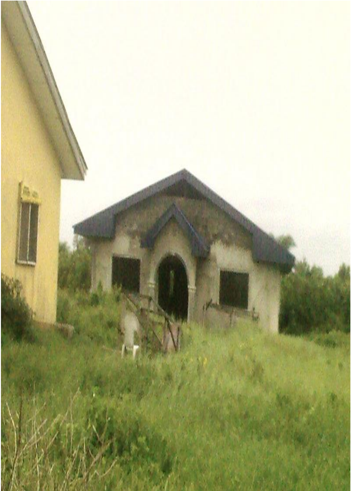
Plate 4.13: Abandoned NDDC town hall project in Ogulagha Kingdom. Source: Fieldwork, 2017
