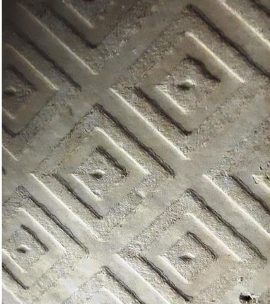
Plate 3.10: Sampled asbestos ceiling
