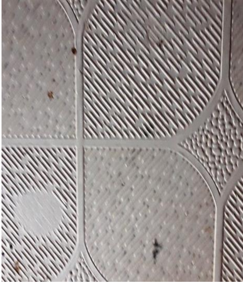
Plate 3.12: Sampled gypsum ceiling
