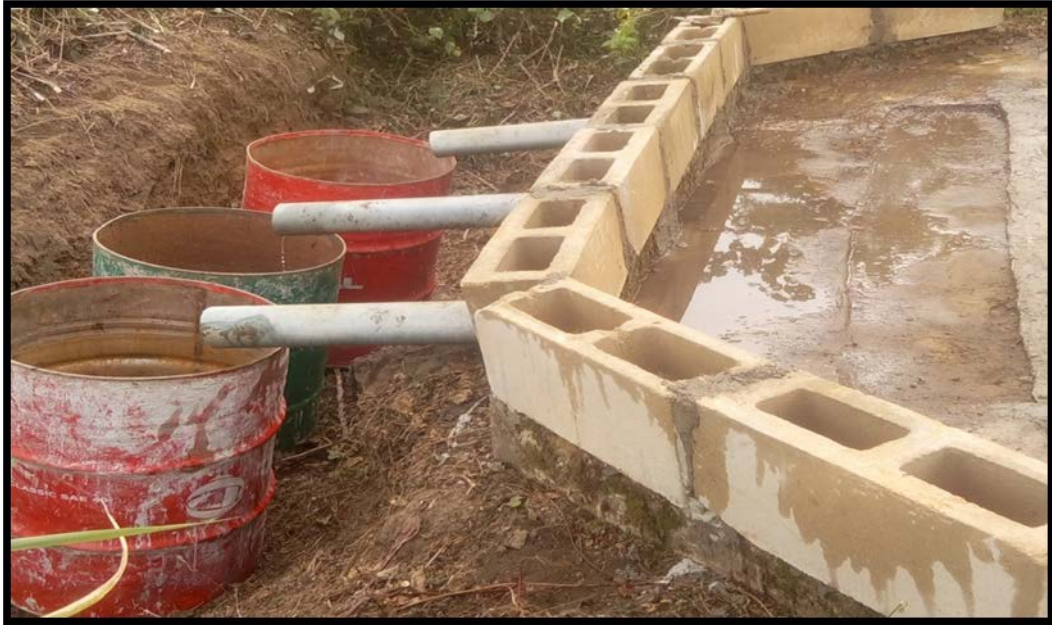
Plate 3.2. The PVC-pipes that channelled runoff to the drums at the downstream of the reseach plot
